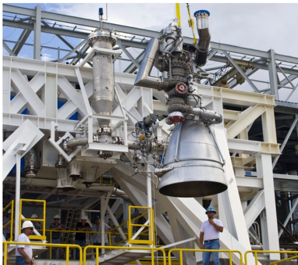
An Aerojet AJ26 rocket engine is prepared to be installed in the E-1 Test Stand at Stennis Space Center.
